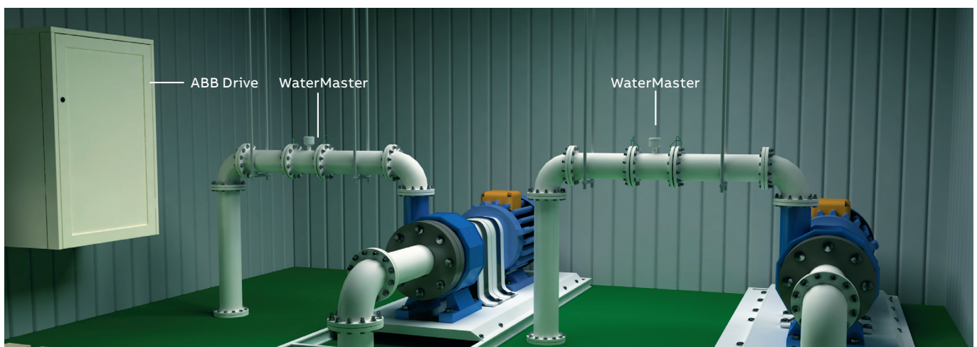
Electromagnetic flowmeters such as ABB's WaterMaster offer long term accuracy and high performance in pumping station applications.
